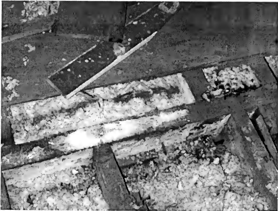
Figure 26 Header for second generation Stair in Attic of the Center Section of the Main House, 2002
